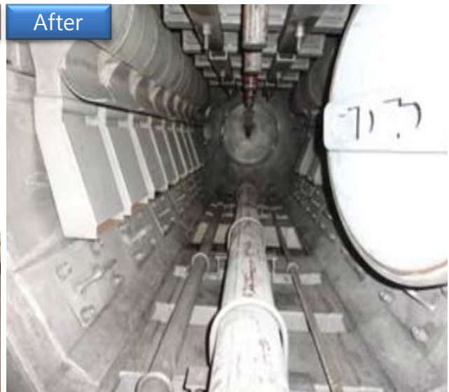
After chemical cleaning Steam Drum
