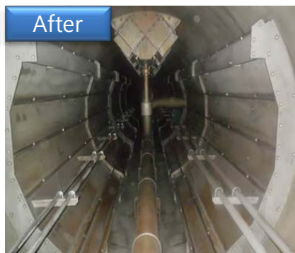
After chemical cleaning Steam Drum
