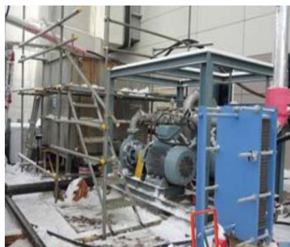
Pump Station Circulating Pump
