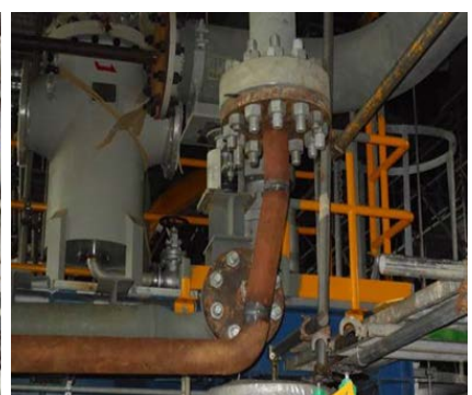
HP BFP Discharge line connection pipe
