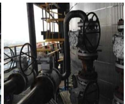
Temporary piping Adsorbent chamber bed line
