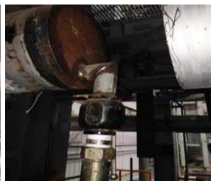
Temporary Piping HP Steam Bypass
