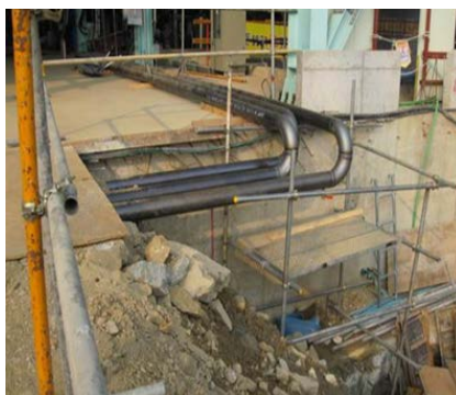
Temporary piping Main circulation line
