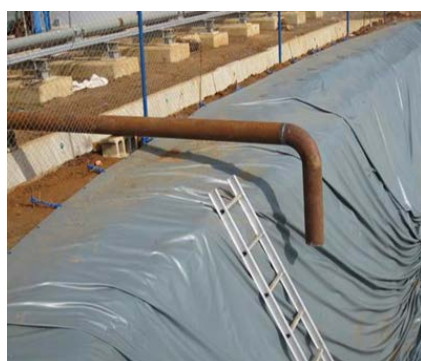
Waste water transfer piping
