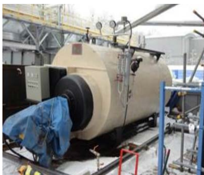
Pump Station Steam Boiler
