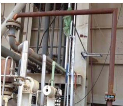
Temporary Piping HP BFP Supply Line
