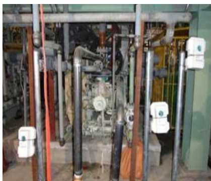
Temporary Piping BFP LP&HP Supply Line
