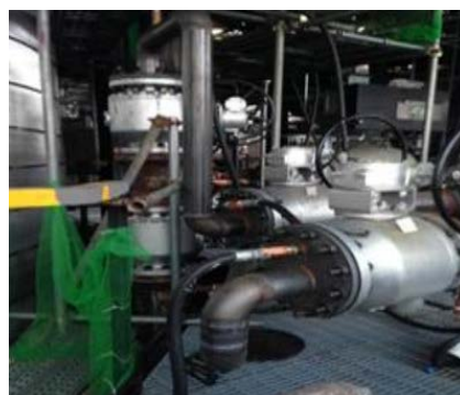
Temporary piping Adsorbent chamber bed line
