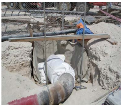
Pig Launcher Ras laffan, Qatar
