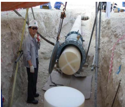
Pig Launcher Ras laffan, Qatar
