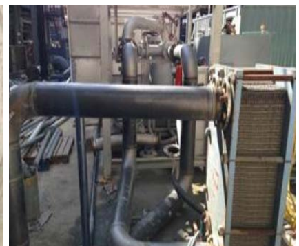
Temporary piping Pump station
