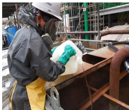
Liquid detergent(NP-10) injection
