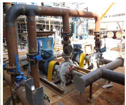
Temporary piping for pump
