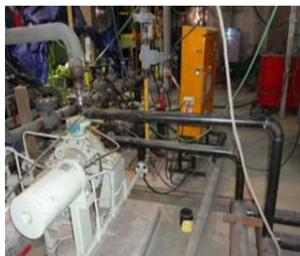
Temporary Piping CPH Supply & Return Line
